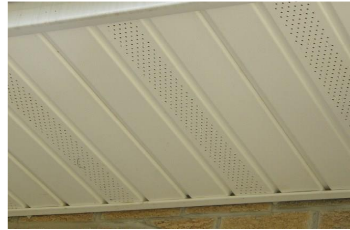
Soffit Panel Vents
