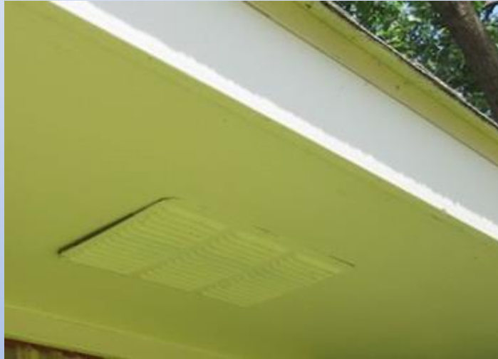
Painted over vents
