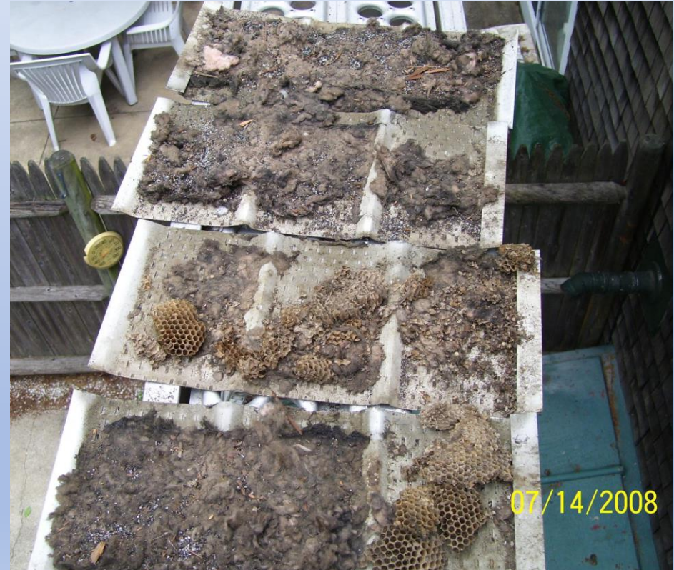
Clogged with debris
