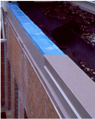
Photograph 1—Excellent Water Management: Notice the membrane under the coping. Notice the slope to the interior. And, notice the drip edges.
