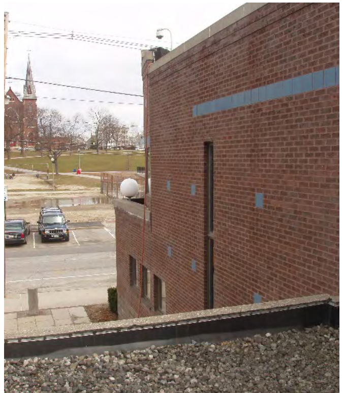
Photograph 3—Membrane Shrinkage: Notice the roofing membrane being pulled away from the cant strip.
