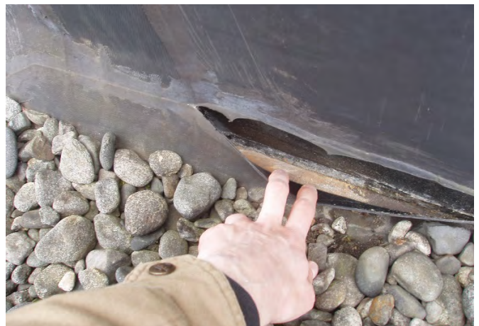
Photograph 4—Tear in Membrane: Membrane shrinkage results in the membrane pulling apart.
