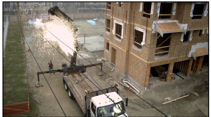
(©WorkSafe BC—Workers' Compensation Board—used with permission)
