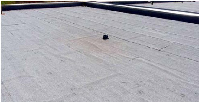
Result of shear and temperature gradient differences (Canadian Roofing Contractors Assn. Photo)
