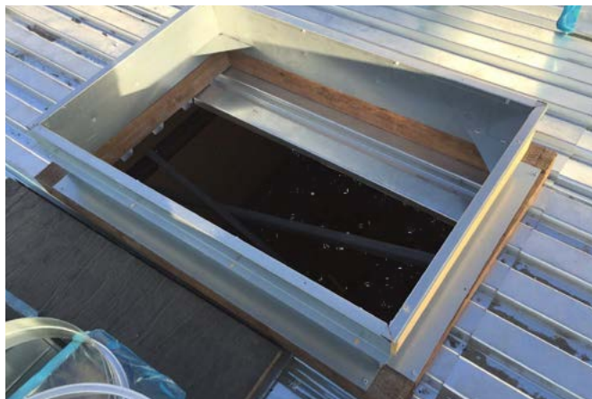
Curb Cut in and Left Uncovered After Accident
