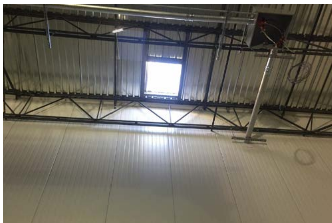
Unsecured Roof Opening Where Roofer Fell Through
