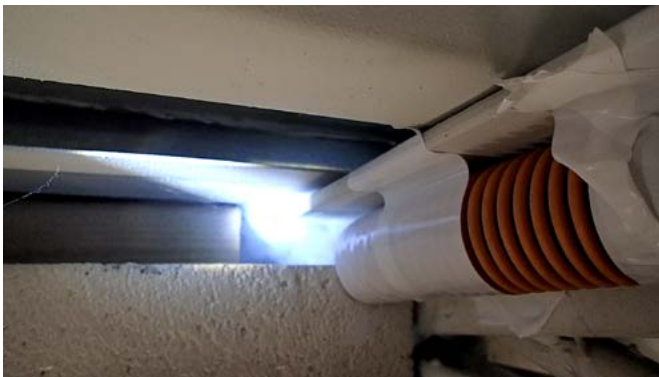
Gaps caused by penetrations of the building envelope to accommodate cables, structural steel, can allow moisture into the building. (SRI, Inc. Photo)
