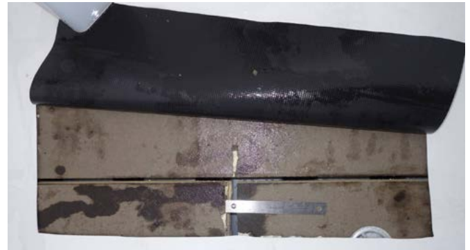
Moisture under roof covering. Note gaps in insulation. (SRI, Inc. Photo)
