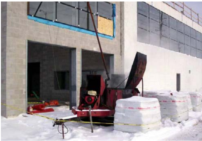
Kettles need to be heated to keep temperatures for application at manufacturer's specs. (Canadian Roofing Contractors Assn. Photo)
